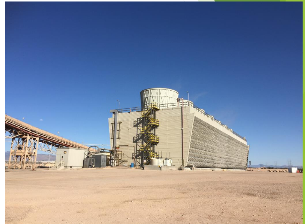
Water Cooling Tower
